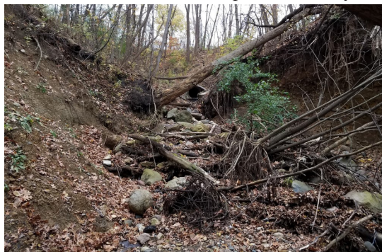
Ravine erosion identified and repaired as part of previous LMRWMO Plan
