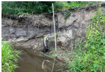
Severe erosion areas along Interstate Valley Creek
