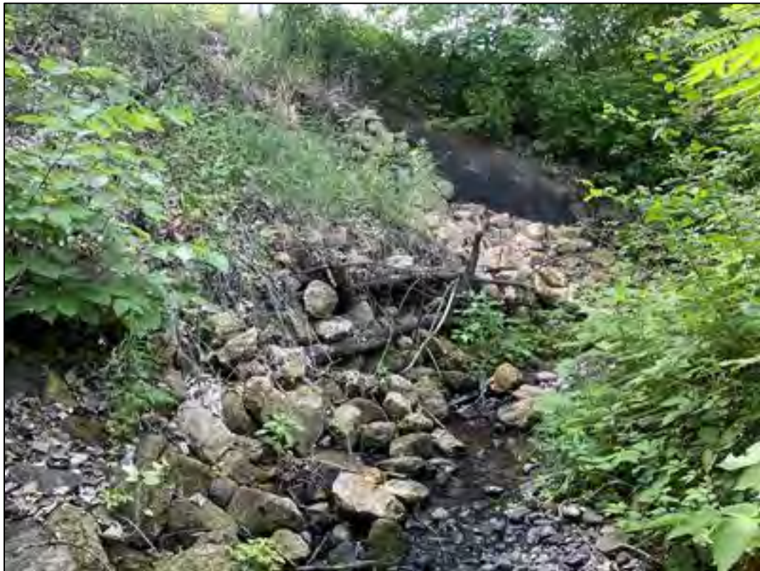
Photo 15: Severe Erosion on Middle Wentworth Creek with Evidence of Past Stabilization Efforts (Riprap over Blanket)
