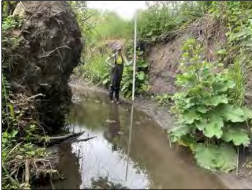
Photo 9: Severe Erosion at Valley Park Wetland Site
