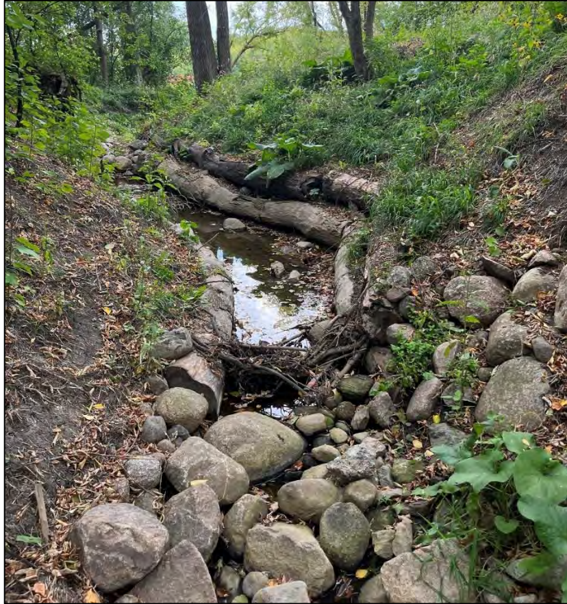
Photo 18: Bioengineered Slope Stabilization in use in Maple Grove One Year Post Installation
