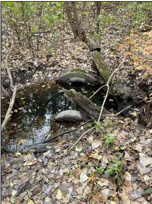
Photo 11: Inlet to Crown Point BMP
