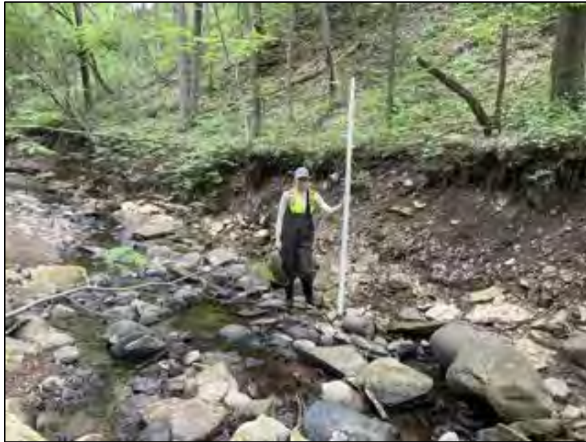
Photo 5: Bank Erosion at Park Place Site
