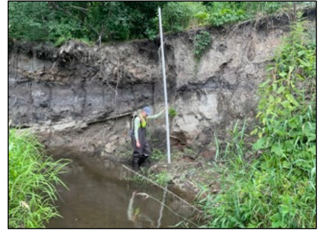
Site 1 – Eroding banks up to 14 feet in height
