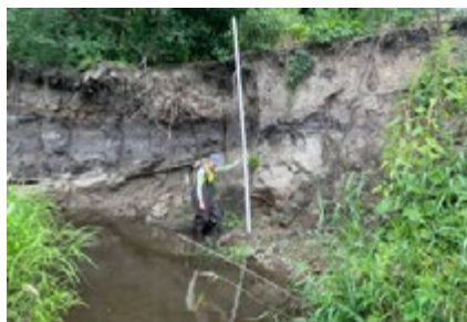
Severe erosion areas along Interstate Valley Creek
