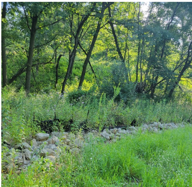
Photo 25 - Existing erosion control at downstream end of I-Strate Trucking Pond receiving ravine
