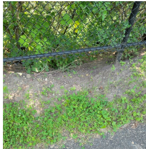
Photo 23 - Minor trailside erosion along Mississippi Regional Trail inside Pine Bend Bluffs SNA.
