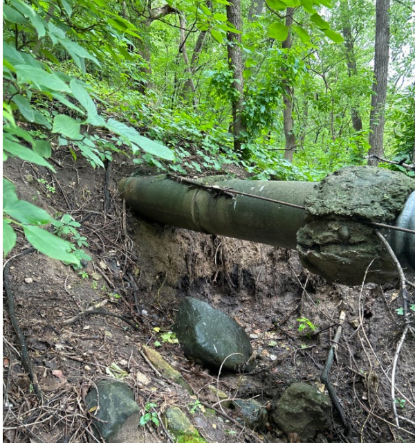
Photo 10 - Leaking structure at Overlook Apartments
