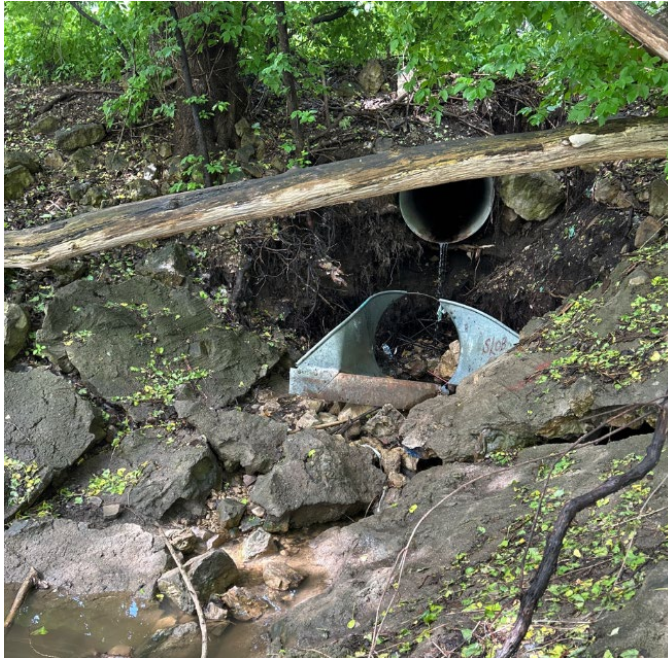
Photo 16 - Damaged outfall to Mississippi River at Kaposia Landing
