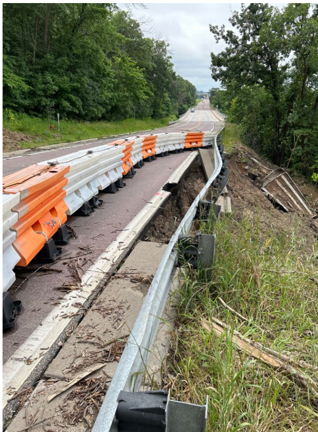
Photo 8 - Highway 13 washout in July 2024
