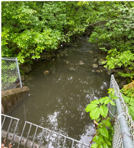
Photo 19 - Existing outfall at top of Dehrer Park ravine
