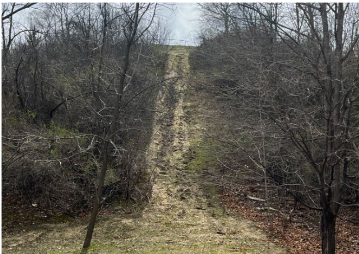
Photo 14 - Photo submitted by City of South St. Paul documenting footpath erosion below Grandview Park
